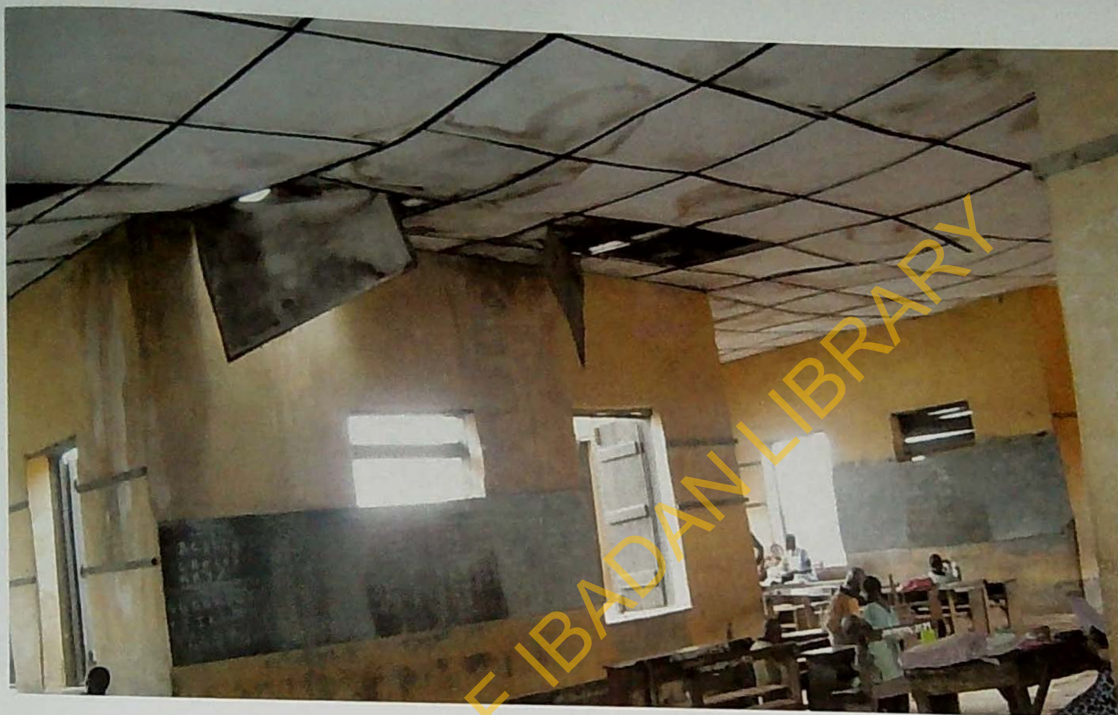
Poor class room condition showing falling roofs, broken windows etc.
