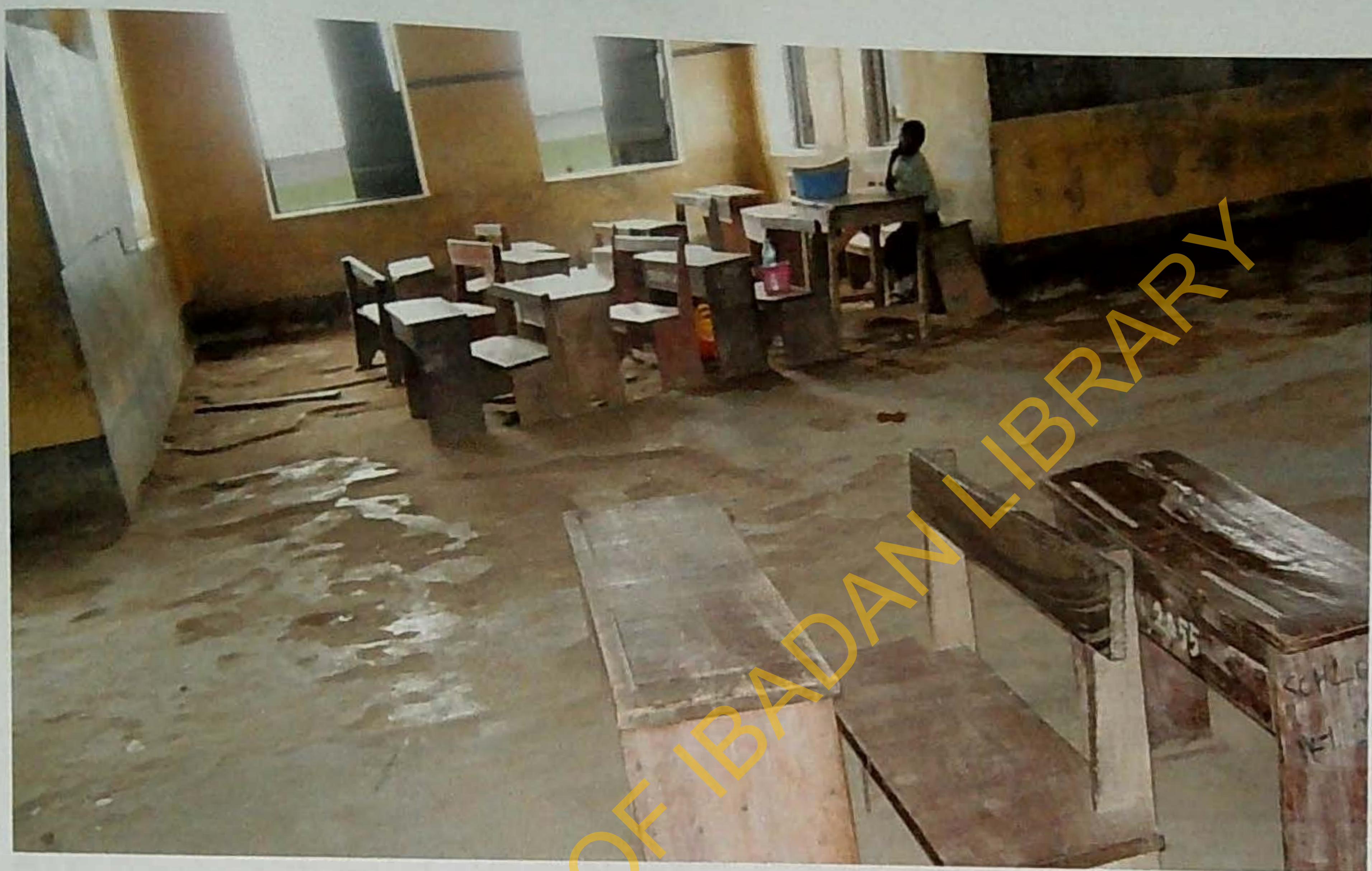
Class room condition showing broken floors/unlevelled ground
