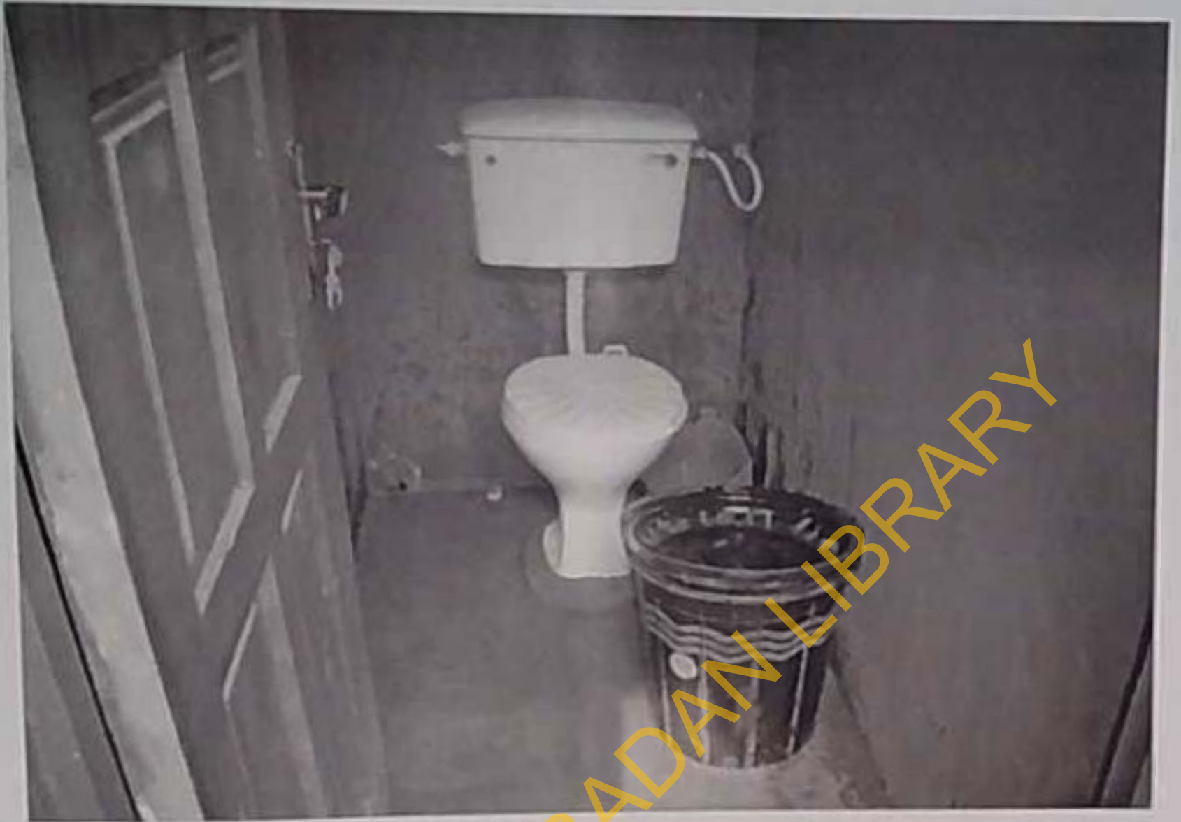
Figure 5.4: Water closet toilet used for toileting in one of the schools
