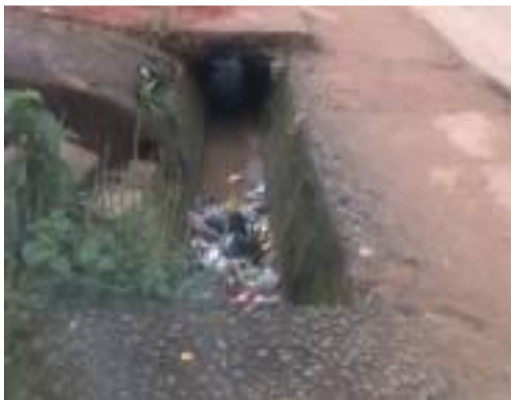
PICTURE SHOWING PRESENCE OF STAGNANT WATER
